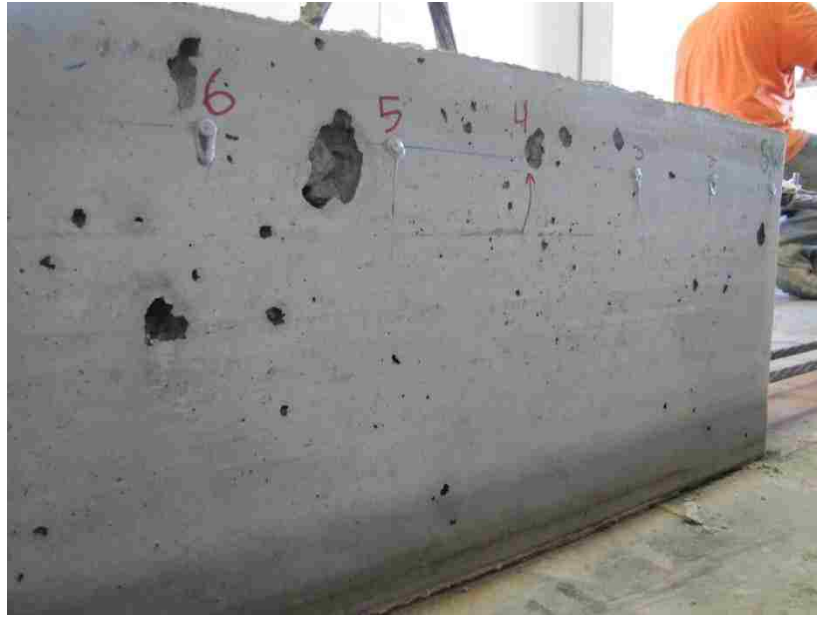
Figure 4.12 – Honeycombing Preventing DEMEC Placement at Point 4 on C10-4-1_SW
